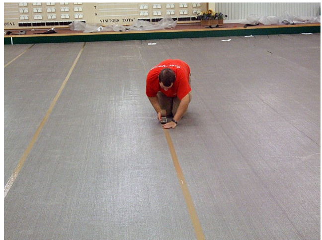
The new underlay is being taped at the seams. This was done with standard parcel tape.
